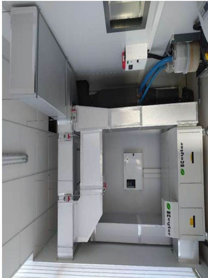
Figure 32: Heat pump and dehumidifiers
